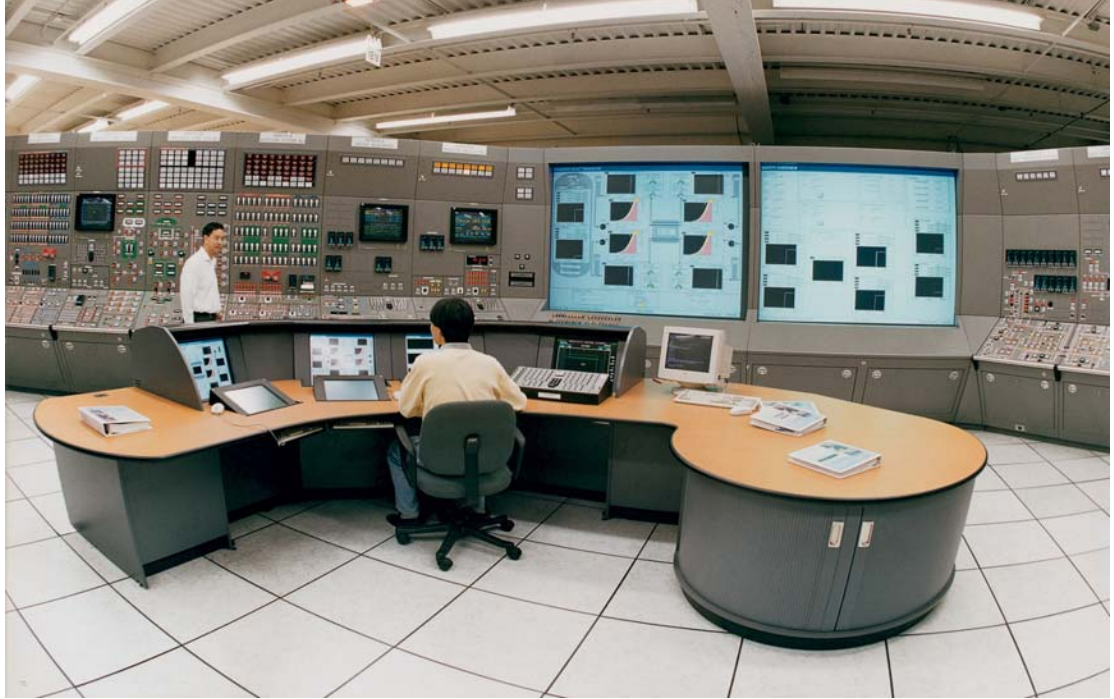
Power System Control Center
